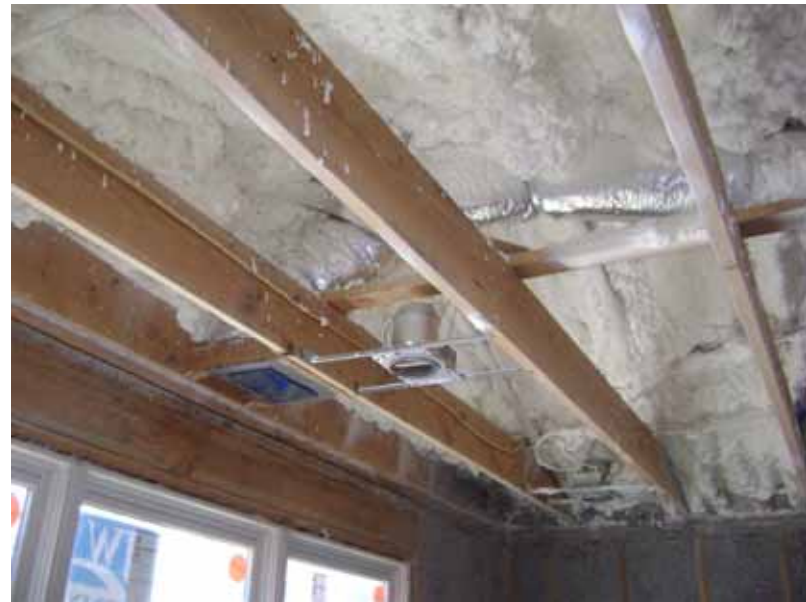
Conditioned Attic w/no attic ventilation
